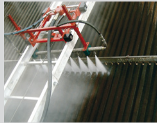
Automated outside cooler cleaning.
